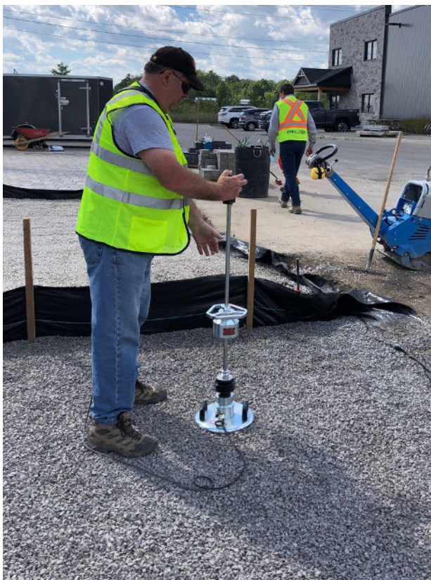
Figure 1- LWD used to verify compaction on the ICP on Open-graded base research project, Fact Sheet 29.
