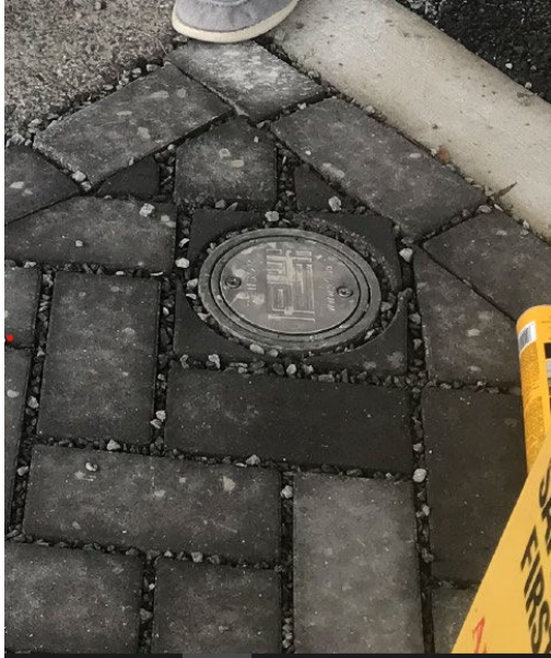
Figure 3: Infiltration monitor installed in the lower PICP parking lot.
