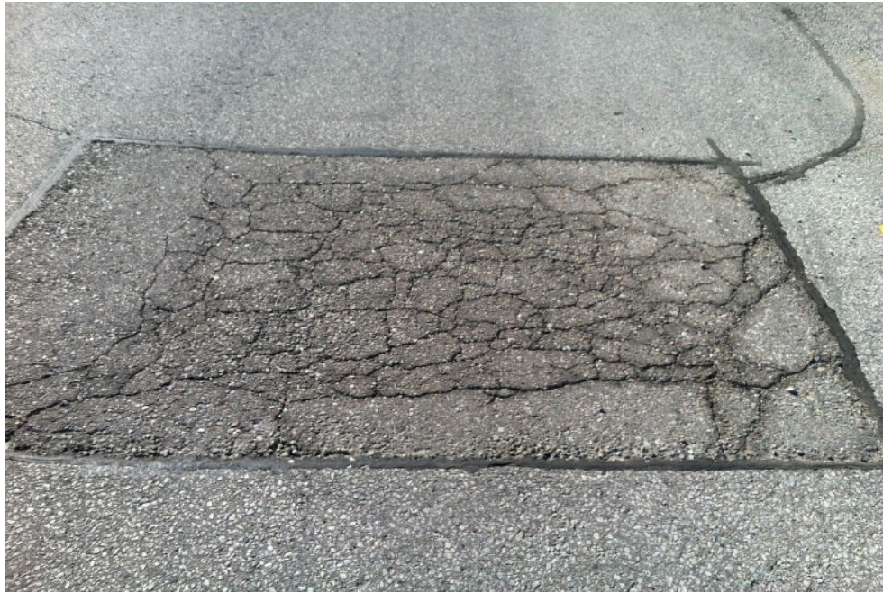
Figure 1-1. Poor Quality Restoration Resulting in Settlement and Alligator Cracking.
