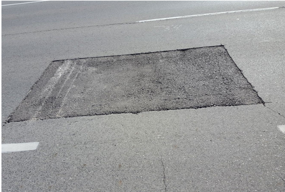
Figure 1-2. Poor Quality Restoration Resulting in Settlement, Cracking and Asphalt Segregation.
