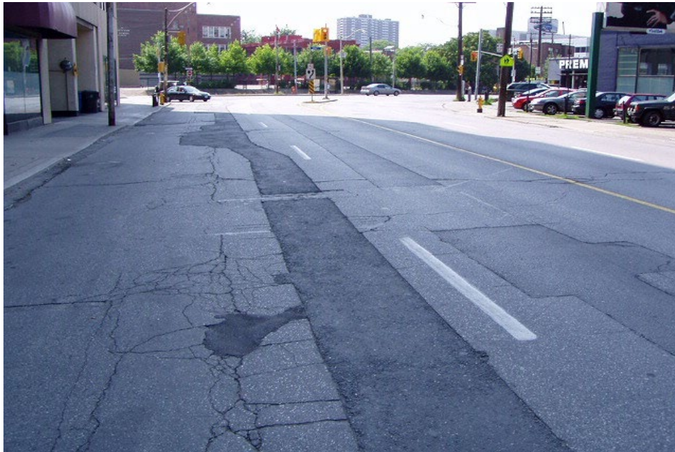
Figure 2-1. Example of an Extensive Longitudinal Utility Cuts.
