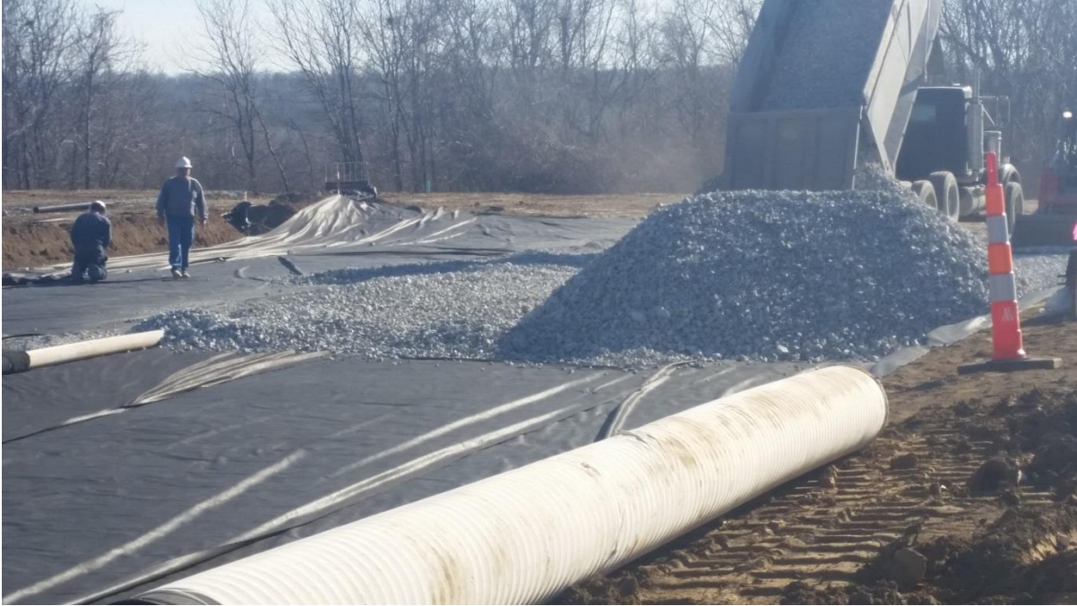
Figure 37. Water Services Base Installation
