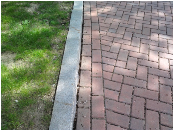
Figure 13: Loss of No. 8 stone along curb line due to erosion and cleaning.
