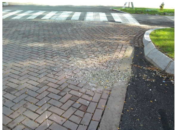
Figure 17: Run on from intersecting MUB drive.
