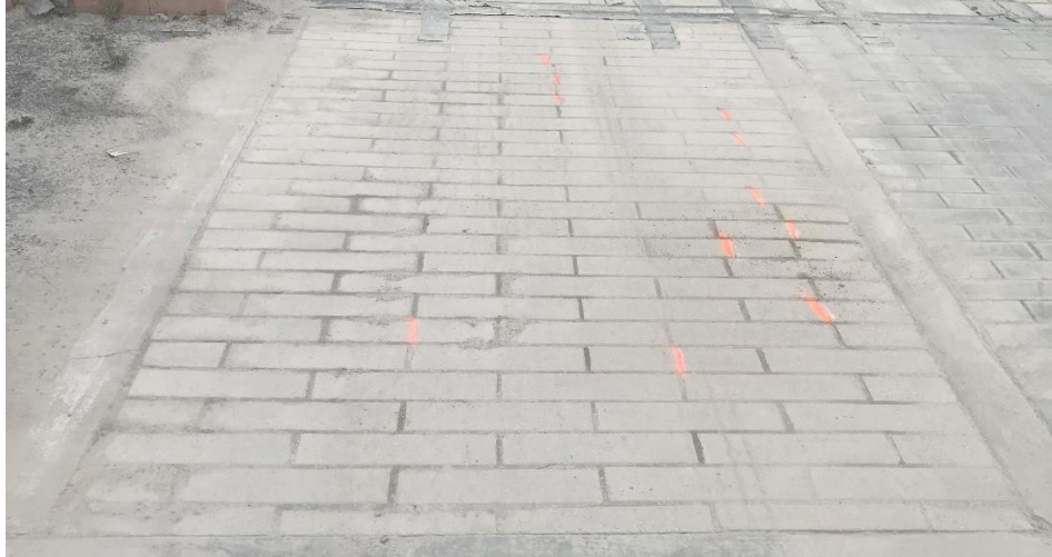
Figure 8: Cell 6. 4 x 16 x 4 in. thick units on a concrete base. Orange paint lines indicate cracks in units.
