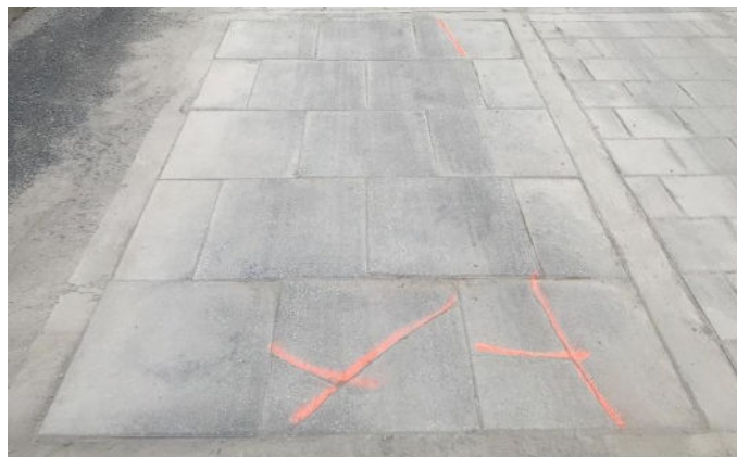
Figure 7: Cell 5. 24 x 24 x 3 in. thick units on a concrete base. Orange paint lines indicate cracked units.
