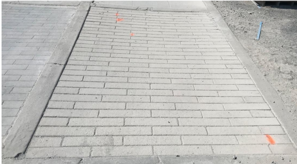
Figure 10: Cell 8. 4 x 16 x 4 in. thick units on an aggregate base. Orange paint lines indicate cracks in units. Picture taken around 30,000 ESALs.
