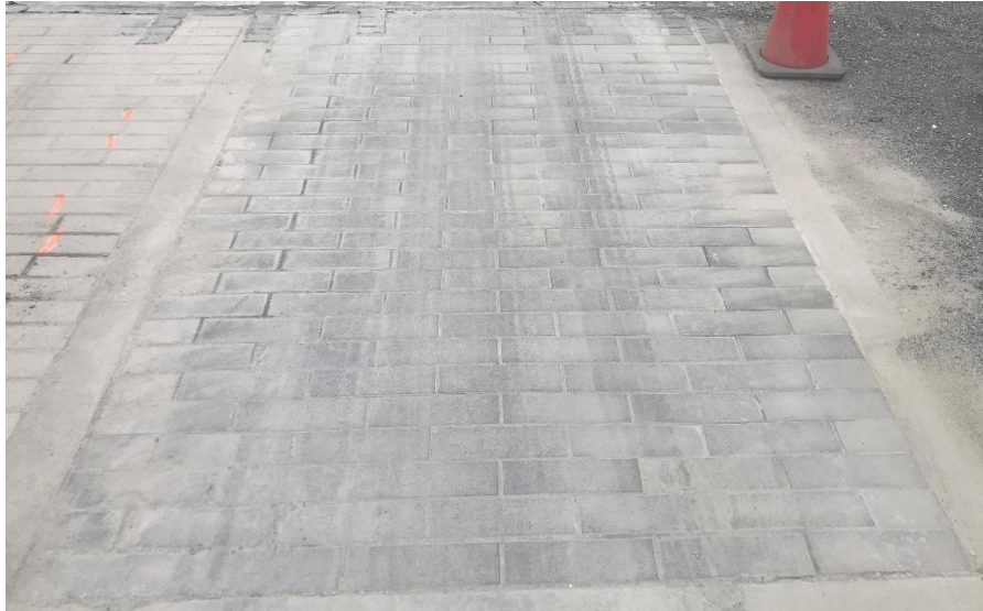
Figure 4: Cell 2. 4 x 12 x 4 in. thick units on a concrete base.
