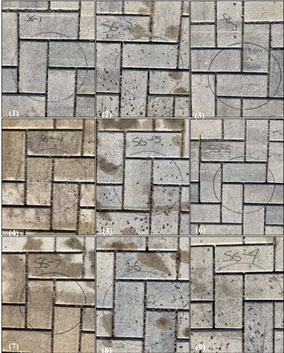
Figure J4. Post-maintenance photos of infiltration measurement locations (1-9) following a regenerative air street sweeper on Cell 6 for second early and repeated maintenance (TYMCO DST-6®).
