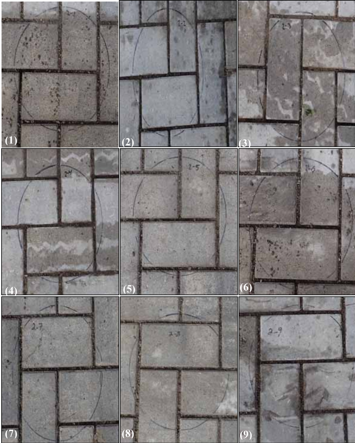
Figure 14. Post-maintenance photos of infiltration measurement locations (1-9) following a regenerative air street sweeper on Cell 2 (TYMCO DST-6®).
