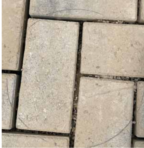
Figure 4-6: Example of sub-surface clay agglomerate left following maintenance
