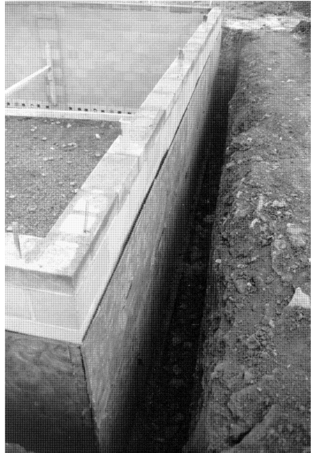
Figure 4-8: Drainage Board Installed On The Exterior Of A Foundation
