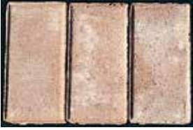
Pavers with efflorescence
