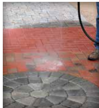
Figure 7. Dry-applied joint sand with a stabilizer is wetted in order to activate it and stiffen the sand. Once the joints dry, they are stabilized.
