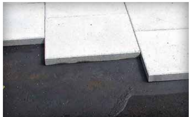
Figure 8. Sidewalk application illustrating the neoprene adhesive on an asphalt bedding layer under paving slabs
