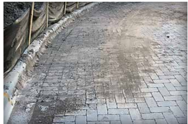
Figure 3. Whether eroded onto or dumped on PICP, erosion and sediment control are essential during construction.
