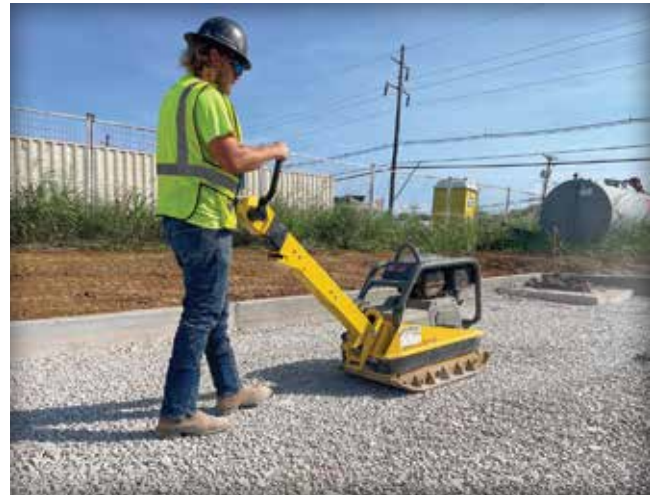
Figure 21. A larger reversible plate compactor is used to compact ASTM No. 57 stone base.
