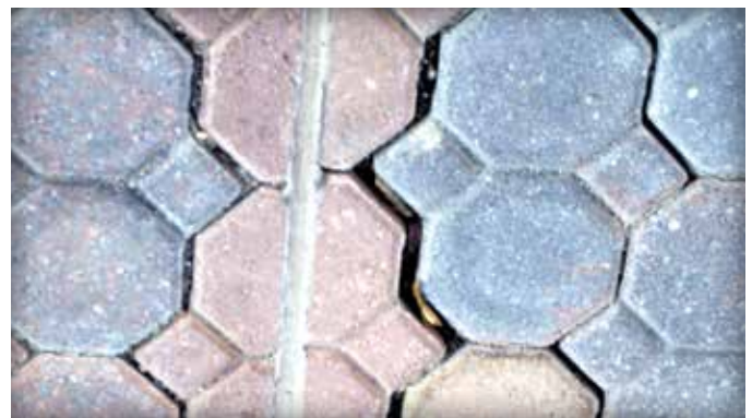
Figure 13. An absence of edge restraints and use of a sealant in this construction joint caused the pavers to shift and open their joints on both sides of the sealant.
