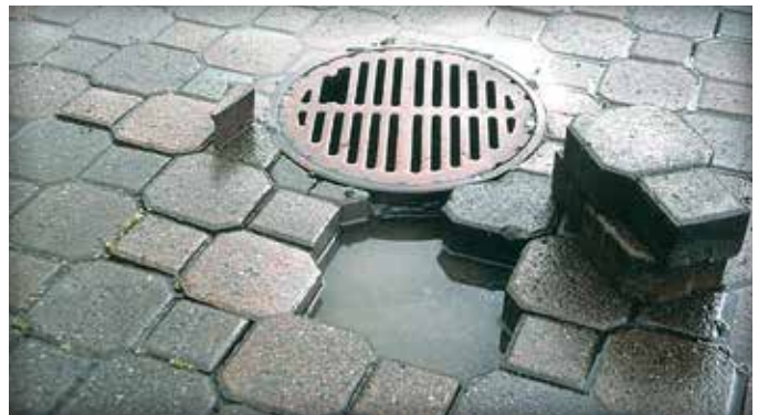
Figure 16. An absence of holes in the sides of this roof drain led to ponding.
