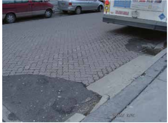
Figure 26. Patching compromises the structural integrity of ICP and occurs when proper maintenance techniques are not followed.
