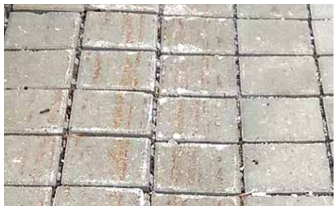
Figure 10. Excessive scratching from a snow plow can lead to rust stains.
