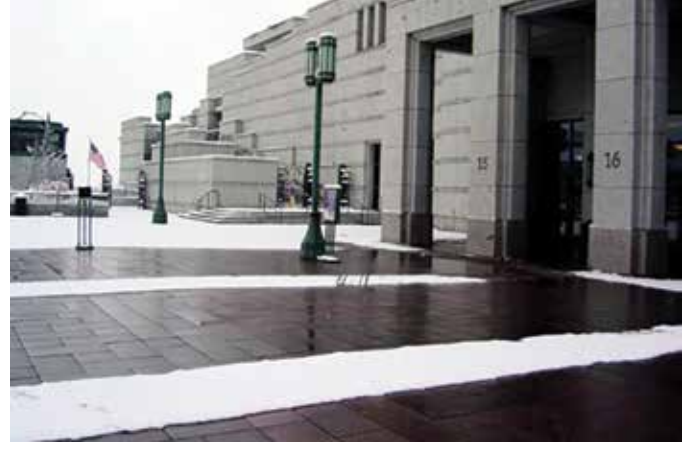
Figure 7. To conserve energy, the snow melt system is only installed directly under the high traffic areas where it is needed.
