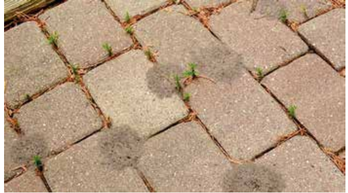
Figure 13. Joint sand stabilization could have been used to reduce the affects of weeds and ants.
