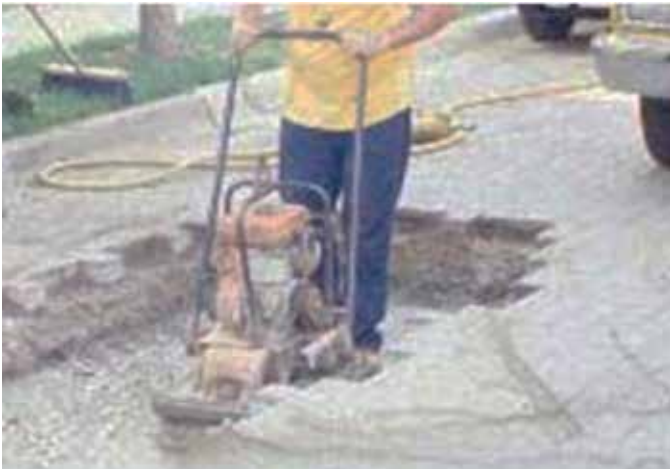
Figure 35. The subgrade should be re-established with a material that can be fully compacted and have little potential for settlement.
