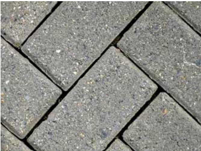
Figure 24. Joint sand loss should be repaired when the void created is greater than 1/2 in. (12 mm).
