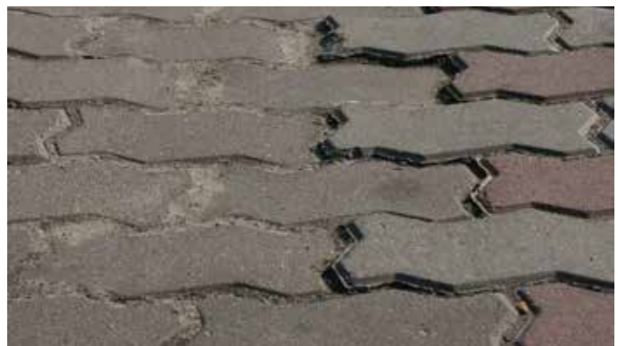
Figure 21. Faulting can be seen as a line of pavers being lifted above the neighboring units.
