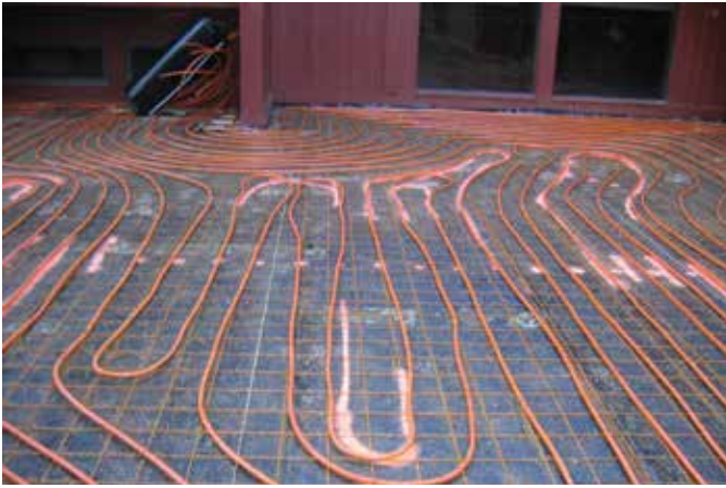
Figure 6. Radiant heating can be installed under the paver surface to melt snow and ice in the winter.
