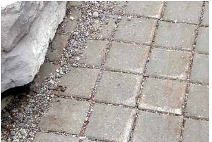
Figure 15. Coarse debris like winter sand should be removed from the paver surface to reduce abrasion.
