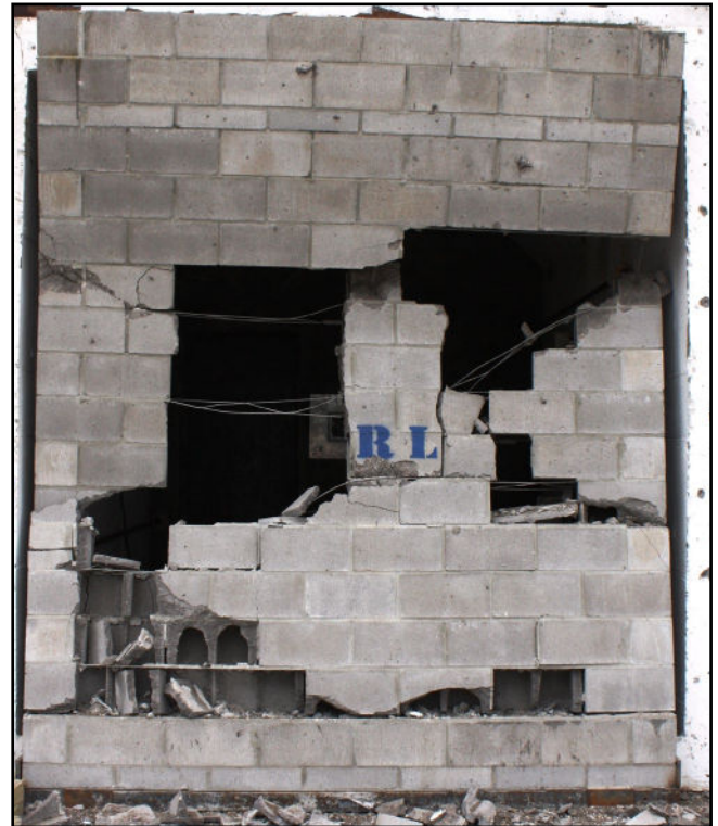
Figure 2—Result of Full-Scale Explosion Testing of Partially Grouted CMU Demonstrating Breaching Tendency
