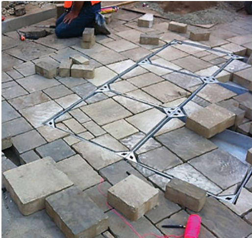
Figure 28. Another example of cutting pavers to accommodate a utility cover set at an acute angle to the paving slab pattern
