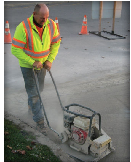
Figure 12. Once the pavers are in place, the joints are filled with dry joint sand and the surface is compacted.
