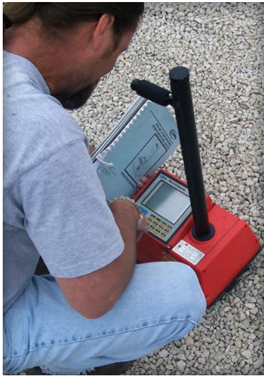
Figure 23. Density testing with a nuclear gauge in backscatter mode can help assess consistent density of the ASTM No. 57 base layer.
