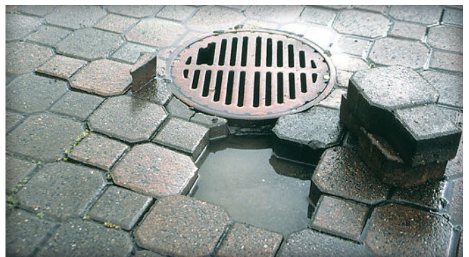
Figure 16. An absence of holes in the sides of this roof drain led to ponding.
