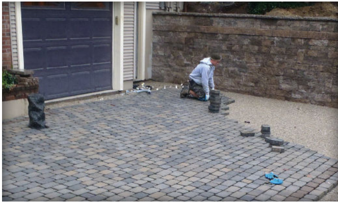
Figure 11. Concrete pavers installed to accommodate permeable bedding and jointing materials, all supported by a permeable stone base.
