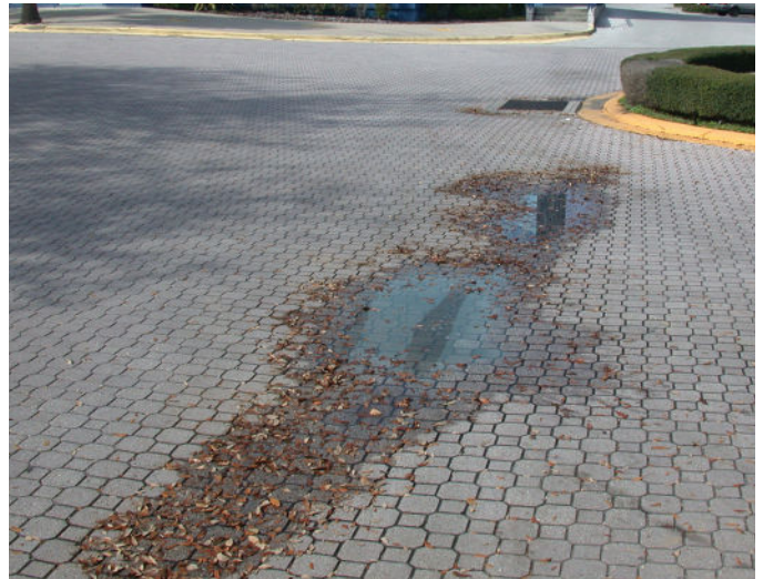
Figure 18. Depressions are caused by settlement of the base or subgrade and are easily spotted by the puddles formed after rain events.
