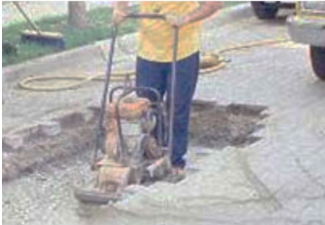
Figure 35. The subgrade should be re-established with a material that can be fully compacted and have little potential for settlement.
