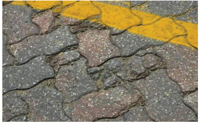
Figure 17. Damaged pavers can be caused by excessive movement of the base or excessive concentrated loads applied to the surface.
