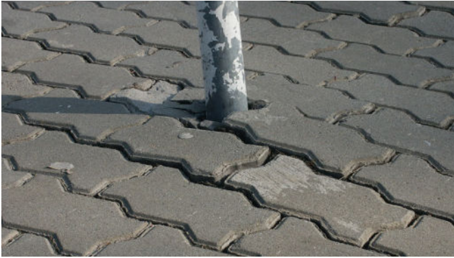
Figure 22. Heave is typically seen near structures that have moved due to freeze-thaw action.
