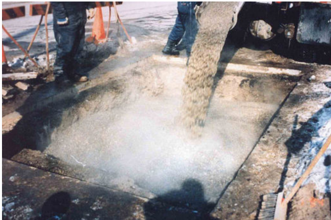
Figure 37. "Flowable Fill" can provide a subgrade or base with little potential for future settlement and not require compaction.
