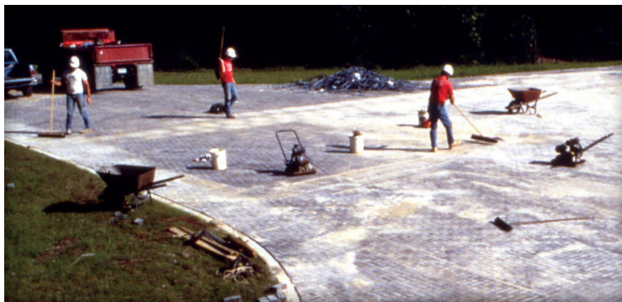
Figure 12. Removing excess sand from the finished surface will make the pavement ready for traffic.
