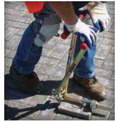
Figure 11. During initial compaction, cracked pavers are removed and immediately replaced with whole units.
