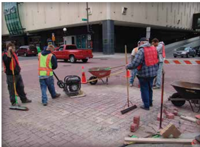
Figure 15 and 16. Reinstated pavers leave no ugly patches nor do they weaken the pavement.
