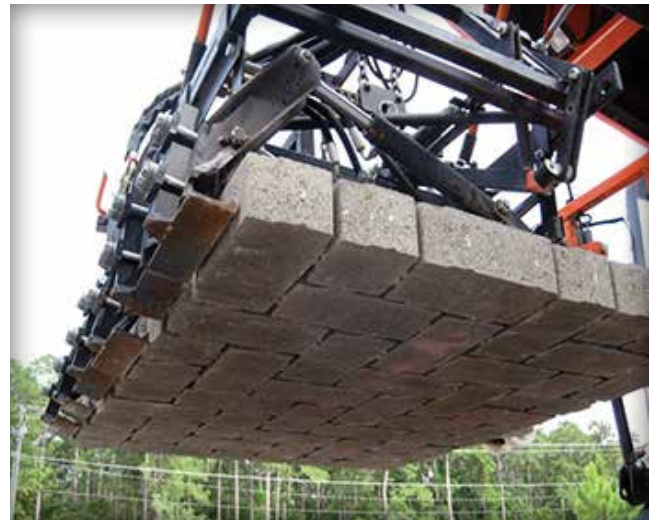
Figure 3. A cluster of pavers (or layer) is grabbed for placement by mechanical installation equipment. The pavers within the cluster are arranged in the final laying pattern as shown under the equipment.
