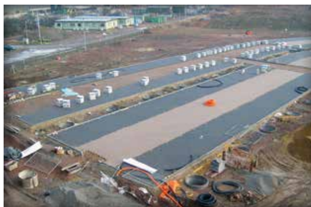
Figure 1-13. The pipes are under a 70,000 sf (6,500 m 2 ) PICP parking lot just completing construction.
