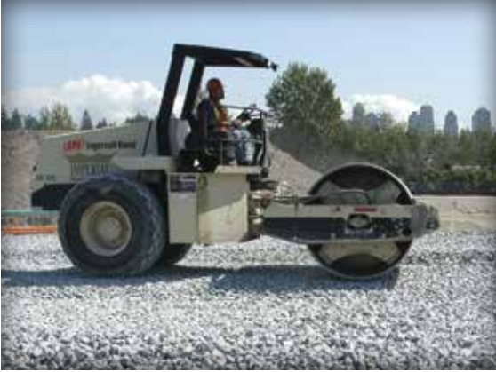
Figure 4-7. A 10 ton (9 T) vibratory roller compactor settles ASTM No. 2 stone subbase for a large shopping center parking lot.
