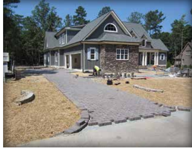
Figure 4-21. An aluminum edge restraint with geogrid is used on this residential driveway.
