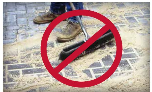
Figure 5-1. Sand-filled joints and bedding common to interlocking concrete pavement are not used in PICP.
