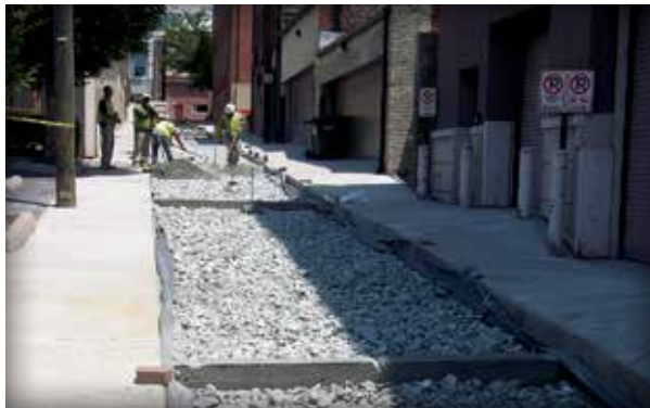
Figure 2-11. Concrete check dams are used to slow flows in this alley in Richmond, Virginia. Subbase and base compaction are critical to minimizing differential settlement.
