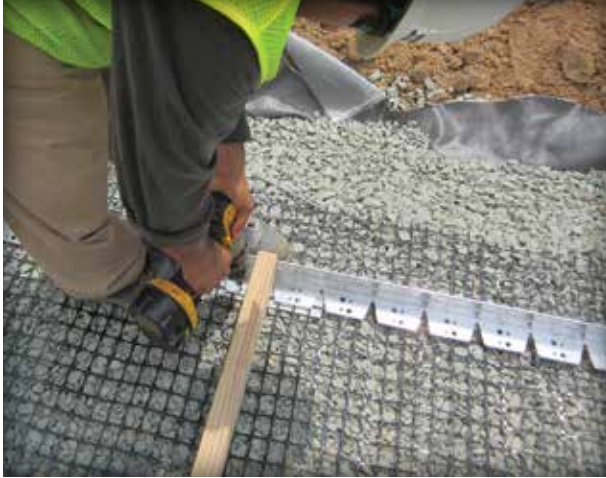
Figure 4-20. Aluminum edge restraint for a walkway is fastened to a geogrid using a separate clamp plate.
