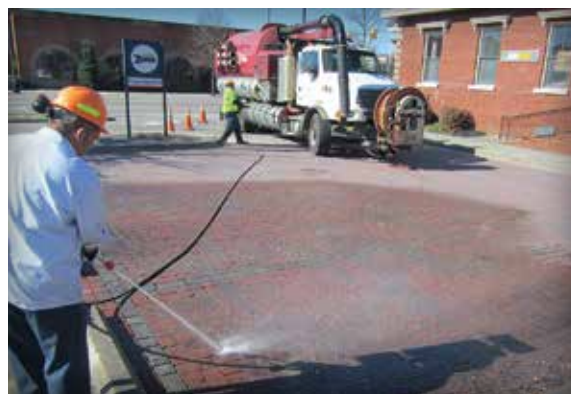
Figure 5-18. Power washing isn't recommended, as it displaces jointing stone and sediment rather than removing it.
