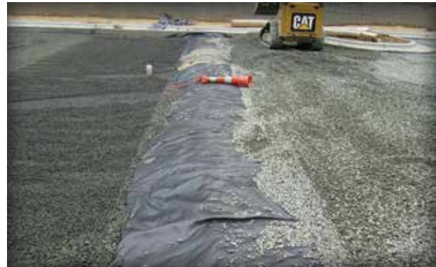
Figure 2-12. Check dams are formed with open-graded aggregate wrapped in an impermeable liner in this parking lot project.
