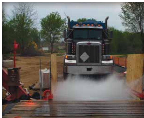
Figure 4-3. Larger PICP projects may require tire washing equipment for trucks to keep mud from contaminating PICP aggregates.
