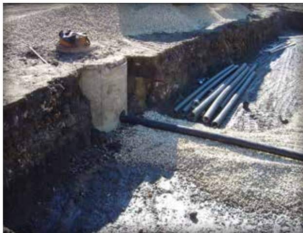
Figure 2-6. Partial infiltration designs typically use perforated pipes raised above the soil subgrade. This enables capture and infiltration of some runoff.
