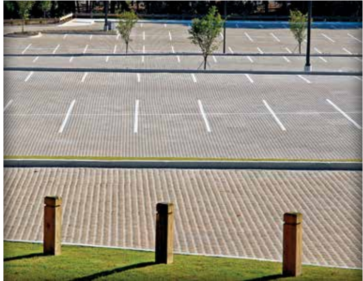
Figure 2-2. A large PICP parking lot manages an overall site slope of 12% using terraced areas.
