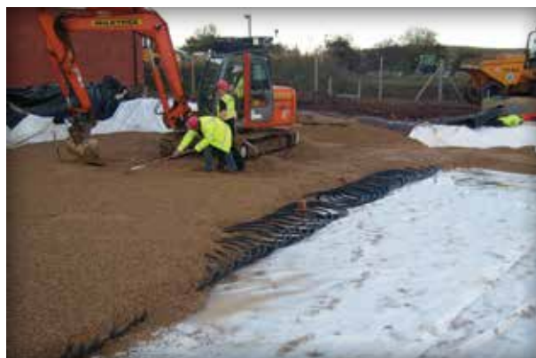
Figure 1-12. Coiled pipes within a PICP aggregate subbase provide heat and cooling exchange for a horizontal ground source heat pump.
