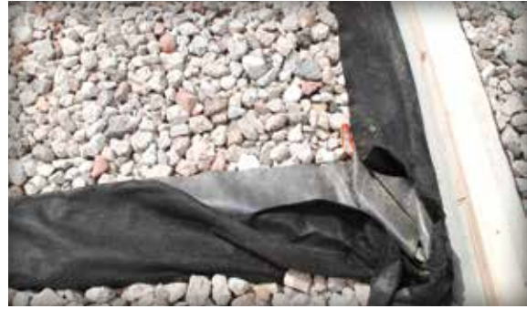
Figure 2-9. The bottom and sides of this PICP subbase are enclosed with an EPDM impermeable liner and geotextile to capture, filter and eventually drain runoff through the subbase via an underdrain.
