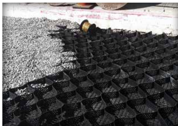
Figure 3-3. Geogrids and geocells are combined for additional PICP support while protecting tree root zones. Geocells were also applied at the bottom of the subbase layer for this street project built on clay soils and subject to substantial traffic.
