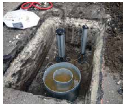
Figure 3-4. A double-ring infiltrometer applied to a test pit measures the soil infiltration rate in preparation for a retrofit PICP street.
