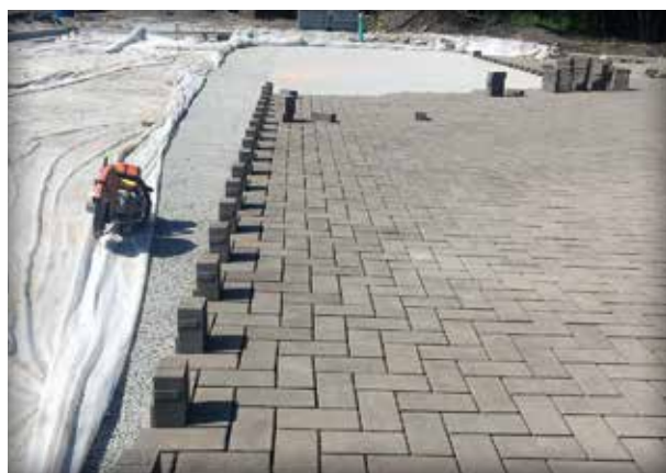
Figure 3-2. Pervious concrete is used as a base under PICP paving units in a Chicago, Illinois, restaurant parking lot. The pavers provide a durable winter surface while the pervious concrete provides improved structural support for heavy trucks. The underdrains lead to the Chicago River.
