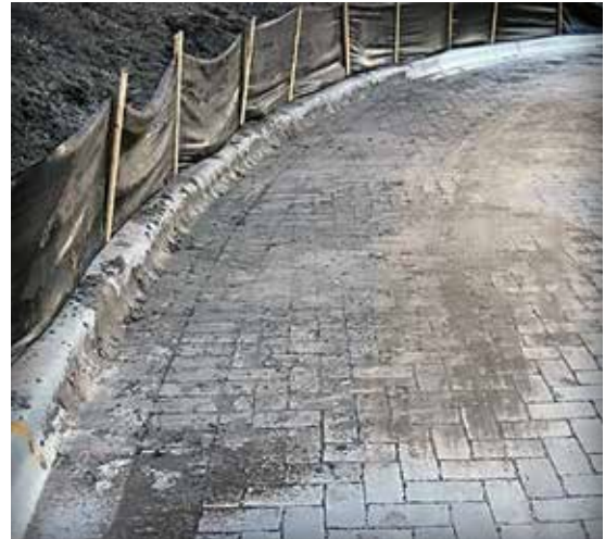
Figure 5-2. Whether eroded onto or dumped on PICP, erosion and sediment control are essential during construction.
