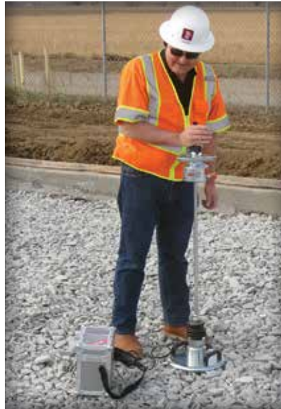
Figure 4-10. Lightweight deflectometer (LWD) testing on a PICP subbase. The device can be used to identify places where compaction was inconsistent.
