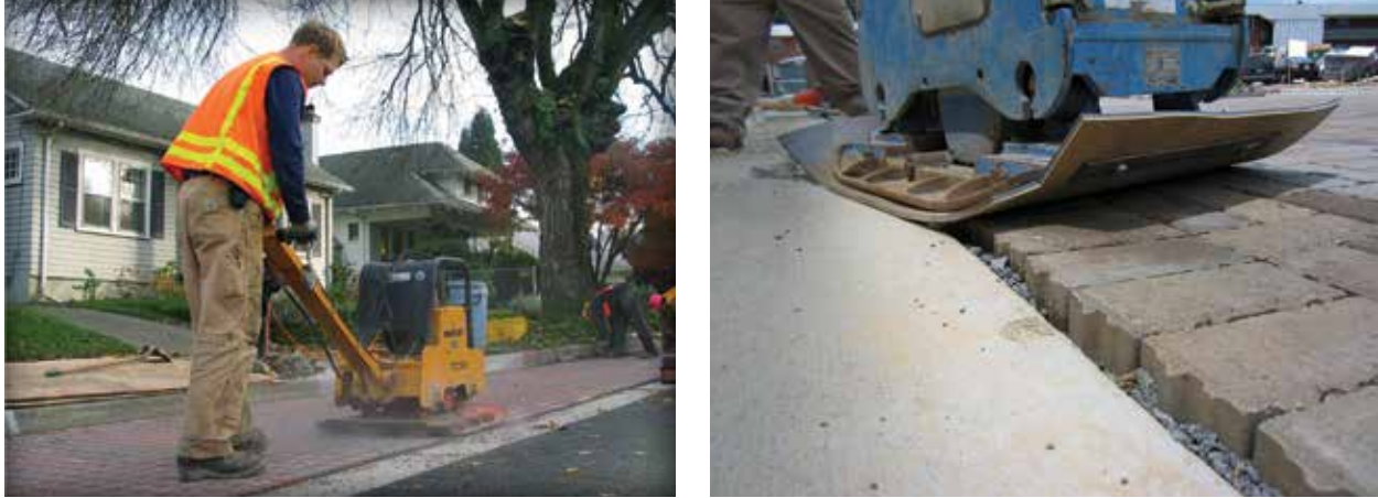
Figure 4-31. Prior to compaction, concrete pavers are typically as set about 1 in. (25 mm) higher than adjacent surfaces or curbs. The right-hand picture shows a pad under the plate compactor to protect the pavers' surfaces from scratches during compaction.
