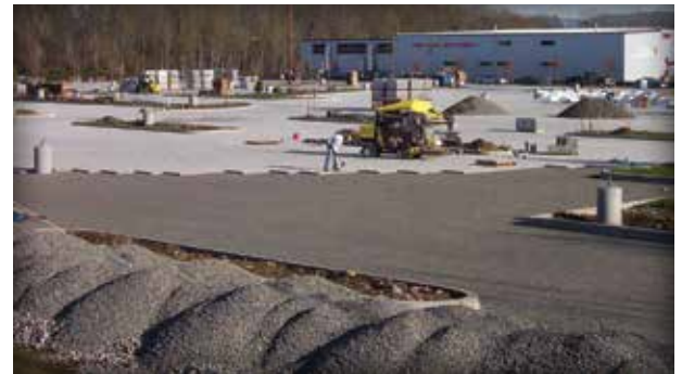
Figure 4-1. Special attention to many details makes PICP construction successful. This mechanically installed project is one of the largest PICP parking lots—about 7.5 acres (3 ha)—at a car dealership in Vancouver, Washington.
