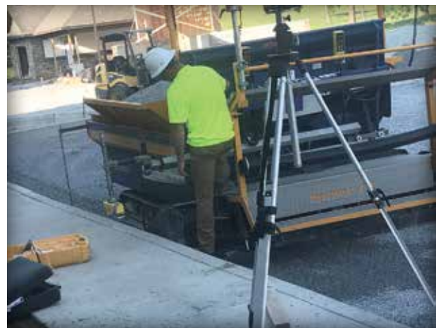
Figure 4-27. An asphalt type spreader specifically designed for spreading bedding stone uses a laser guidance system to keep elevations consistent while spreading.
