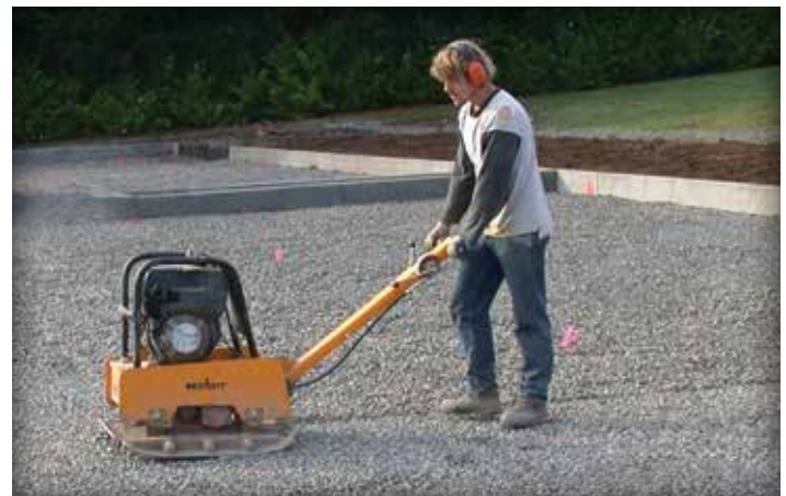
Figure 4-9. A 13,500 (60 kN) vibratory plate compactor is used on this ASTM No. 57 stone base.
