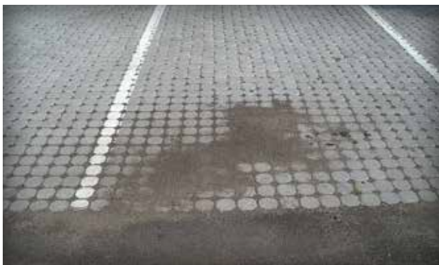
Figure 5-9. Erosion of adjacent asphalt and sediment deposition on PICP.
