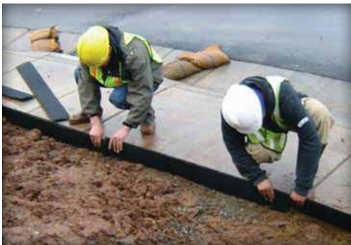
Figure 4-2. This temporary permeable edging around bare soil replaces silt fencing because it restrains sediment while allowing water to pass.
