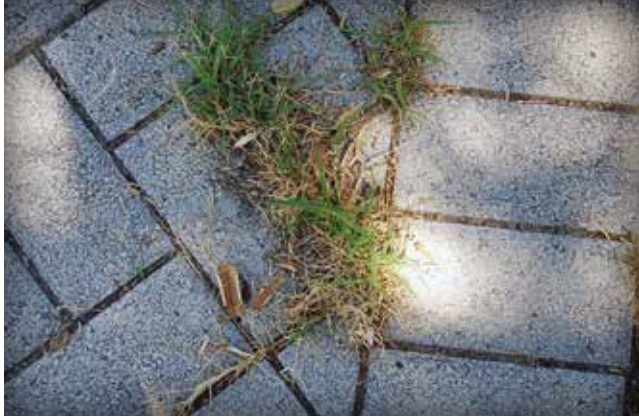
Figure 5-8. Weeds indicate sediment accumulation and lack of surface cleaning to remove it.
