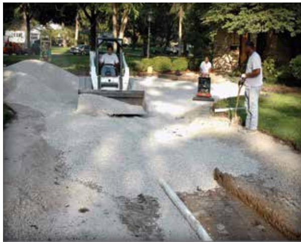
Figure 4-16. Perimeter berms made with dense-graded base are in place prior to placing open-graded aggregate in the driveway.
