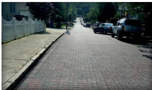
Figure 1-6. Approximately 4 miles (6.4 km) of PICP in SE Atlanta, Georgia, is used for flood mitigation for a more resilient infrastructure.
