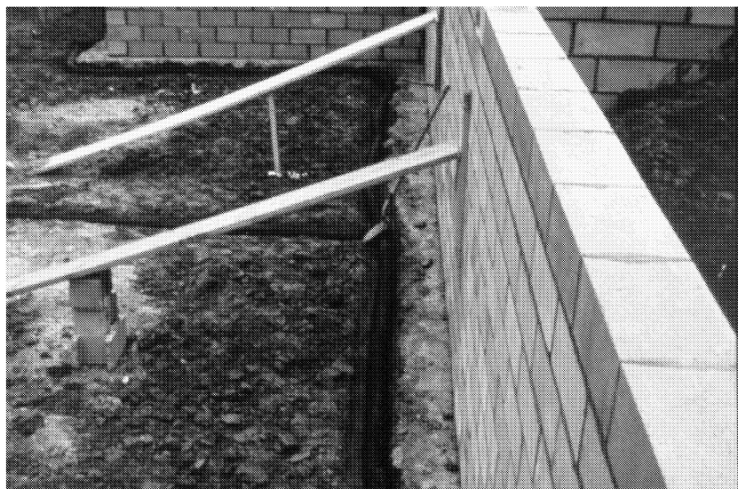
Figure 4-6: Pipe Drainage System
