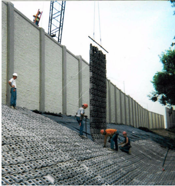
Figure 6—Cabled ACB Installation Behind a Sound Barrier
