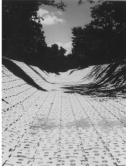
Figure 7.5—Bed and bank protection with minimum radius-of-curvature at grade changes and top-of-slope termination points.
